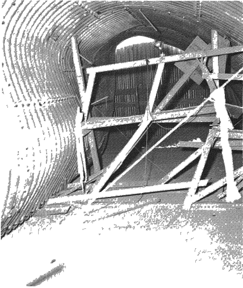
Figure 4 46 Severe damage to earth-covered surface corrugated steel structure will be noted that about half of the arch has collapsed This failure was attributed primarily to the dynamic pressure acting on the forward slope of the earth mound.
